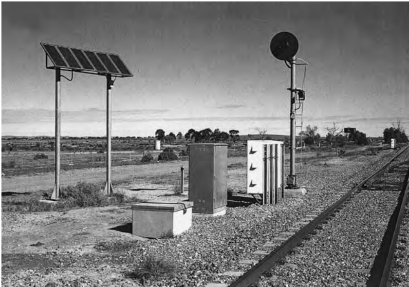
Figure 7.27 A typical stand-alone application of photovoltaics: powering a railway signal box in a remote area of Australia. [Photo by courtesy of BP Solar.]
